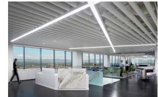
Manage and optimize lighting
