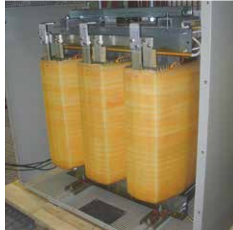
400kVA with aluminium windings
