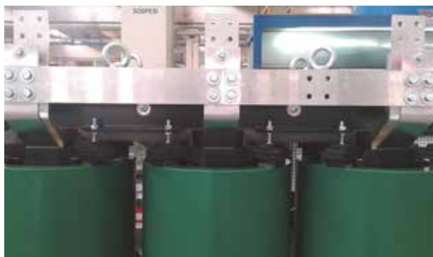
Example of LV terminals
